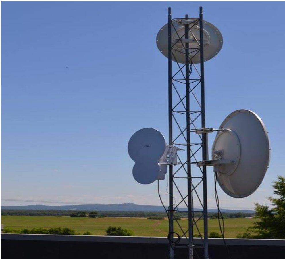
A VABB Tower. Photo credit: Virginia Broadband
