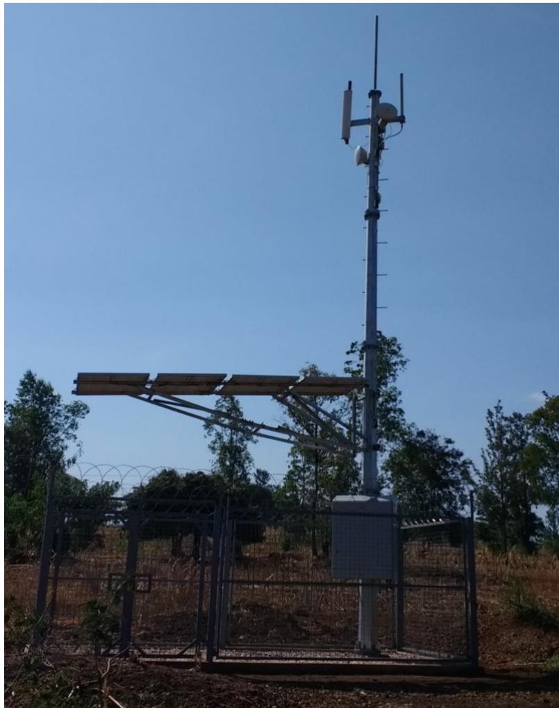
A Vanu tower. Photo credit: 1 World Connected
